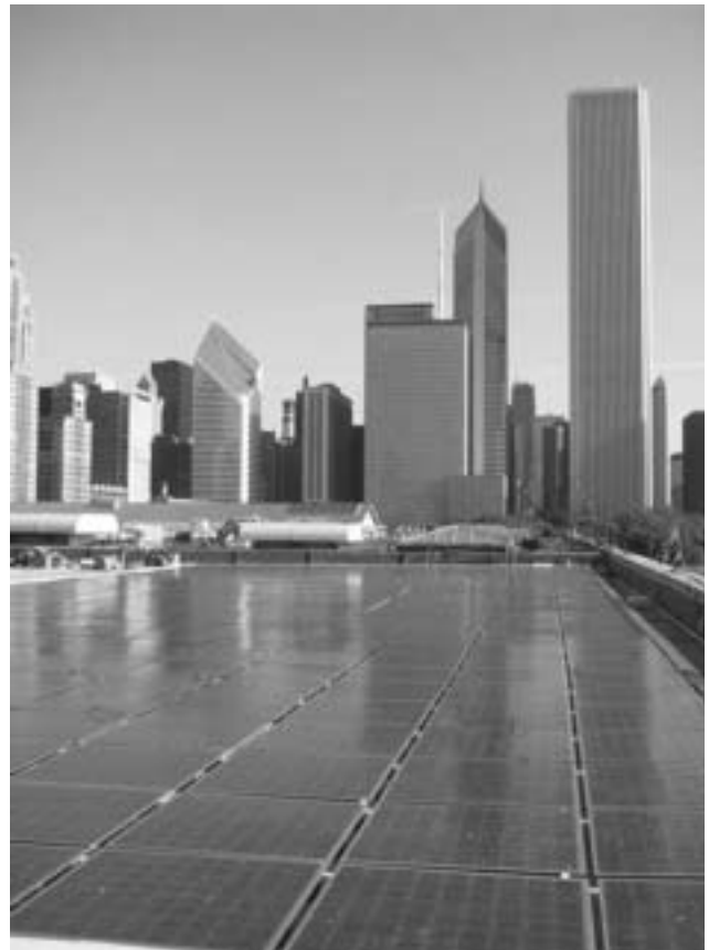
NREL/Spire Solar Chicago
