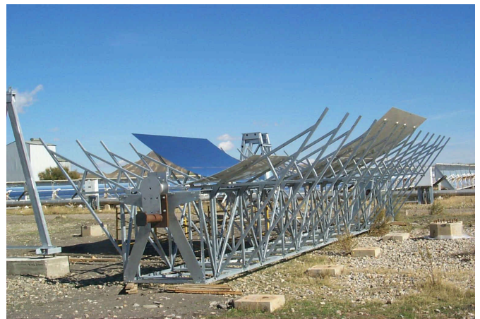
Figure 4: View of the EURO TROUGH support structure taken during mirror assembly.
