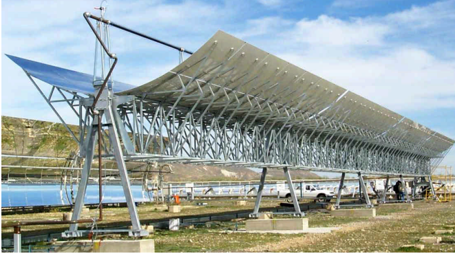
Figure 5: The EURO TROUGH collector prototype tested at PSA has currently four, later six collector elements to one side of the hydraulic drive.
